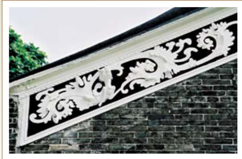
山牆上的草尾灰塑裝飾 Mouldings of leafy patterns in the gable wall
